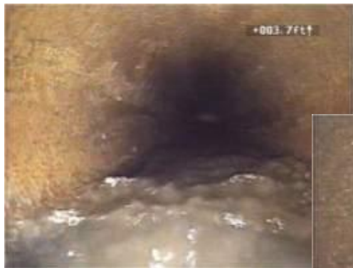
Sag, poor vertical alignment
